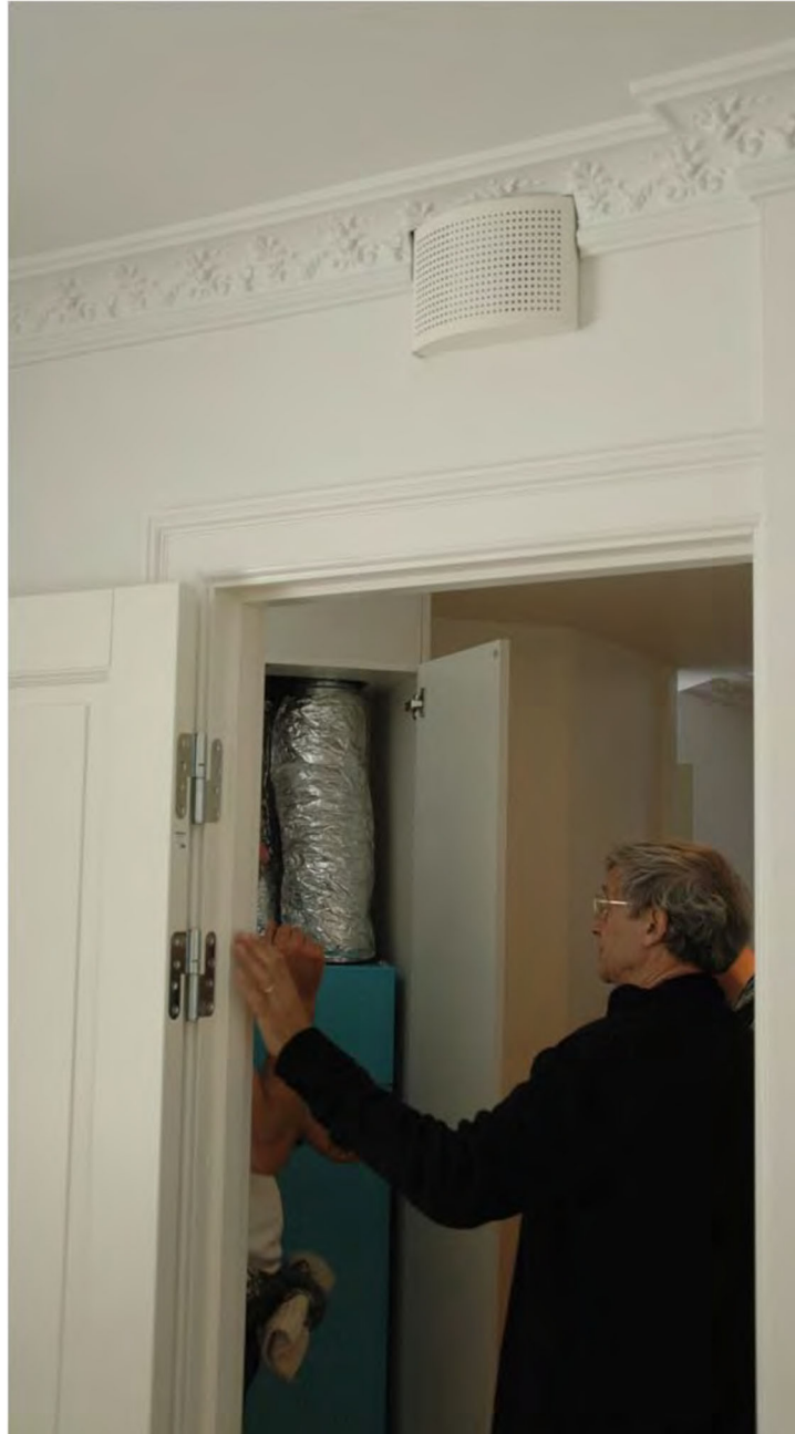
Fig. 2. Decentral ventilation system in a kitchen closet.
